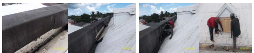
Part of damaged roof before repairs
